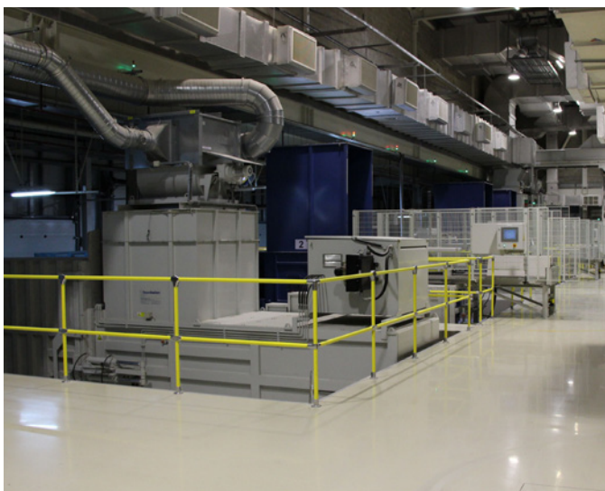
Al Nisr Publishing has fully automated the disposal of printing waste. No manual interference is necessary, from receiving the waste material at each production line to filling the container.
